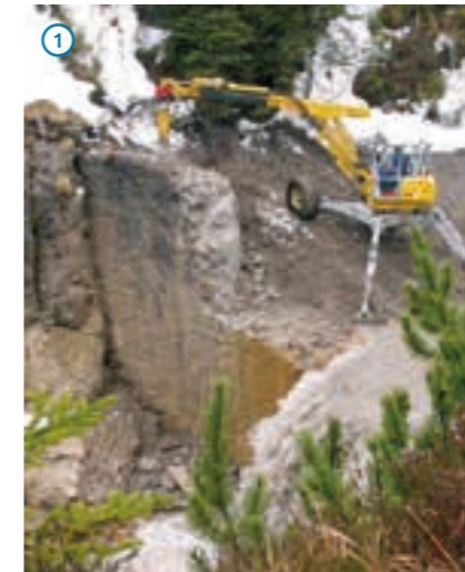
1 Removal of the Hornbach retention dam during the first LIFE project at the Tyrolean Lech 2001-2007
