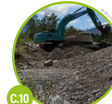
C.10 LECH FORCHACH Groynes were shortened, a channel was reactivated as the “Koppenbach”, and the river area given over to dynamisation. → page 16
