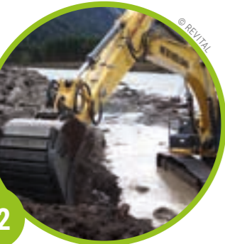
C.1 VORDERHORNBACH “Soft” banks with rich structural diversity replace linear “hard” banks. → page 13
